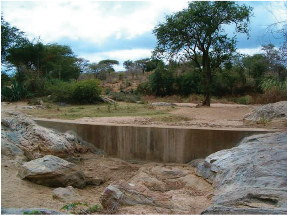
(a) Small sand dam in Kitui district, Kenya. [Photo: Sander de Haas]. The dam has created a small sand reservoir in the stream bed where flood water is stored. This can be abstracted to meet modest local water demands.
